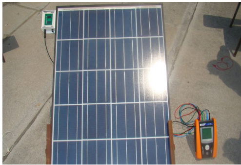
Figure 14. Single module PV system.
